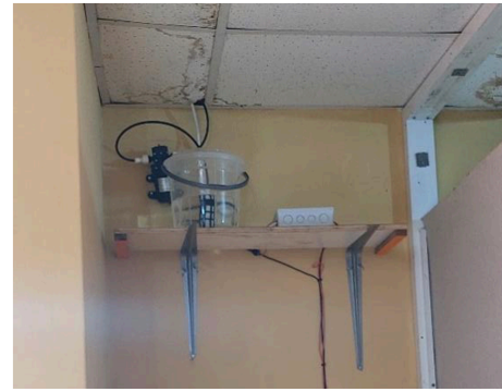
Fig. 9: Pump unit and control unit mounted on a wooden platform inside the building
