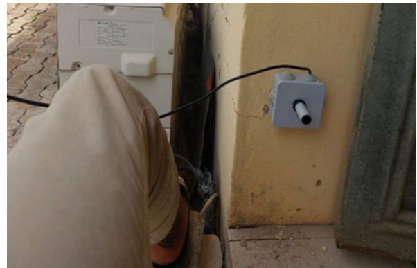
Fig. 6: Mounted Photoelectric sensor (1ft from Ground Level)
