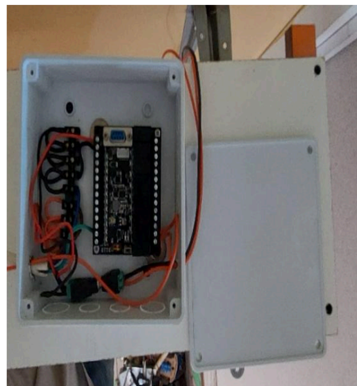
Fig. 8: PLC control unit for the disinfecting system
